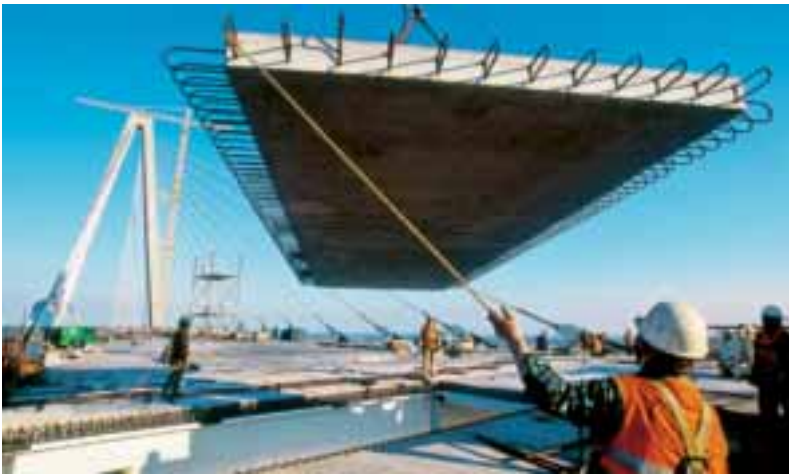
Construction of North America's longest cable stay span, the Cooper River Bridge, which connects the city of Charleston and the town of Mount Pleasant, South Carolina, was completed in spring 2005. Skanska completed the project a year ahead of schedule.
